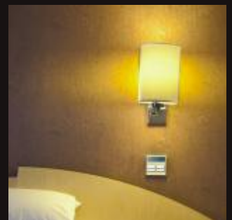
Touch Button Panel for Mood Lighting
